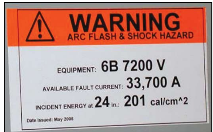
Figure 6. Energy level of 201 cal/cm 2 @7.2K V
