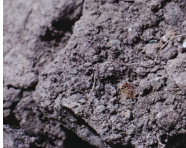
Why test? Corrosive soils.
