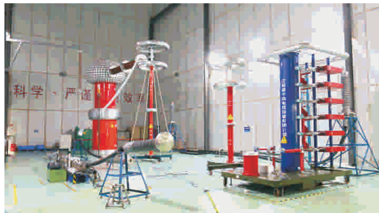
High voltage laboratory
